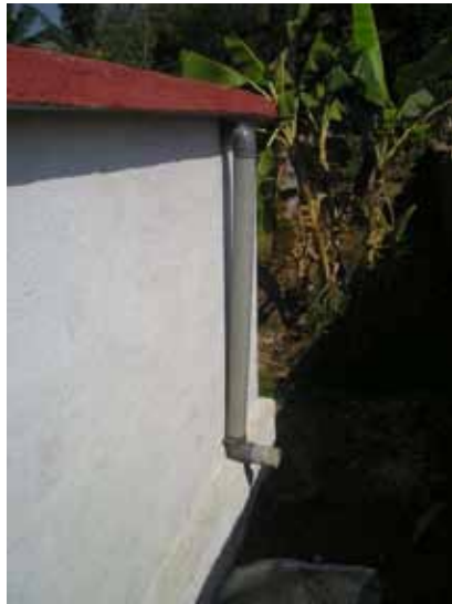
Overflow pipe with mesh
