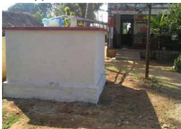
Rainwater storage tank
